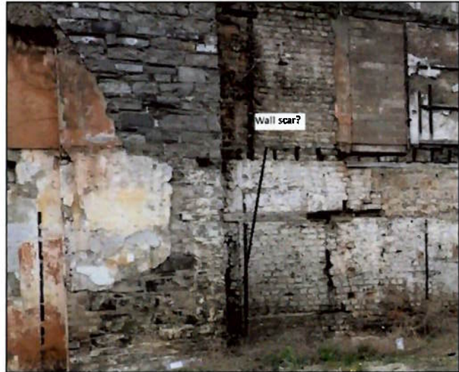
Figure 81 Wall scar of Building 2
